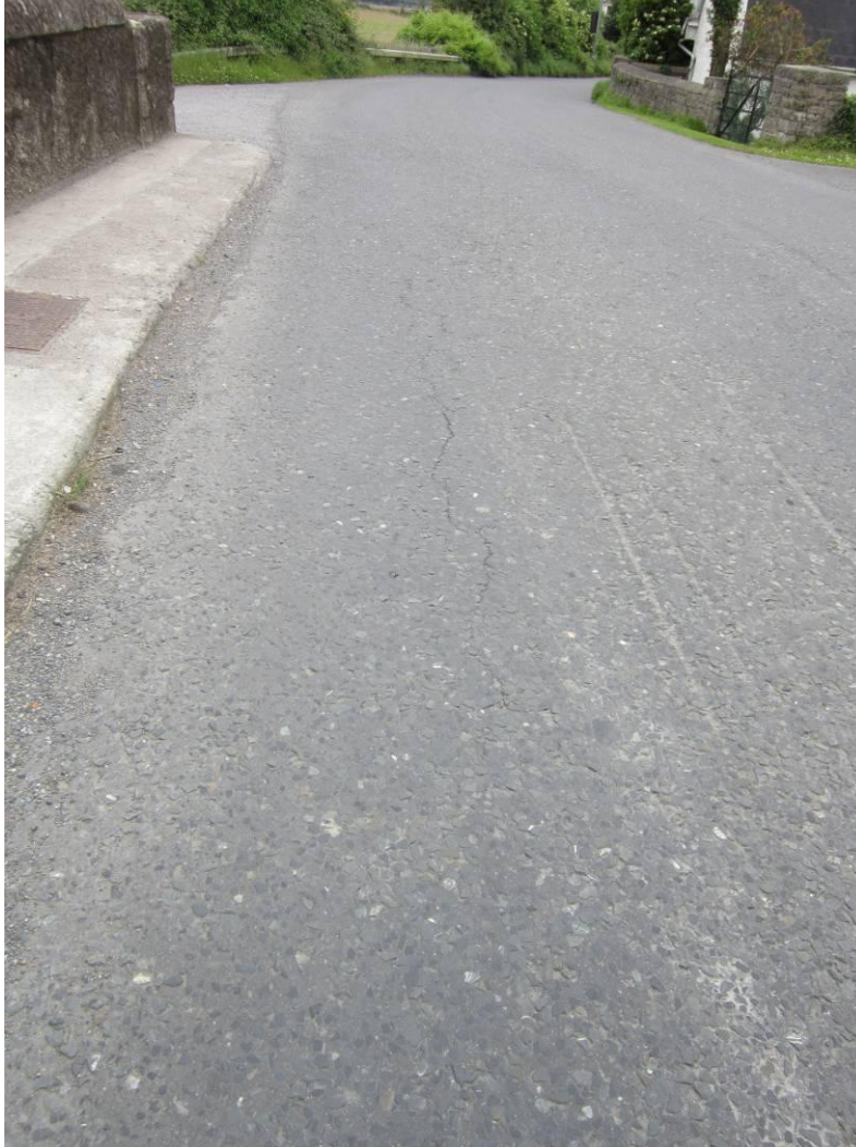
Photograph 3: Longitudinal Crack in Surfacing
