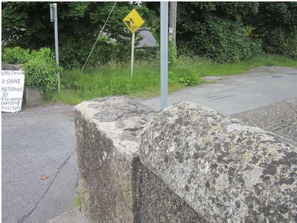
Photograph 5: Missing Granite Coping Block at NE Corner
