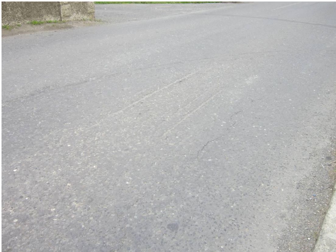
Photograph 2: Gouging at Crown of Arch
