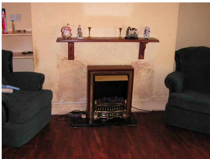
Fig. 7.9. Ground floor of number 3 Millview. Moisture in the base of the chimney stack, probably caused by lack of ventilation of the flue and deterioration of the top of the chimney above. (May 2011)
