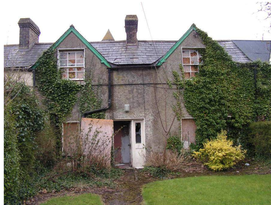
Fig. 7.5. Ivy and weeds colonising the front façade of 2 Millview Terrace. (March 2013)
