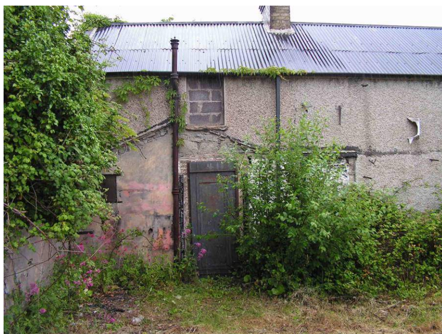
Fig. 7.4. The rere façade of number 1 Millview Terrace. Grasses and weeds have colonised some of the wall tops and the gutters. A shrub is thriving near the base of the rere façade. Note the outline of the pitched roof of the former extension which was demolished about a decade ago. The roof was destroyed by fire and a new corrugated sheet metal and plastic roof installed. (June 2013)
