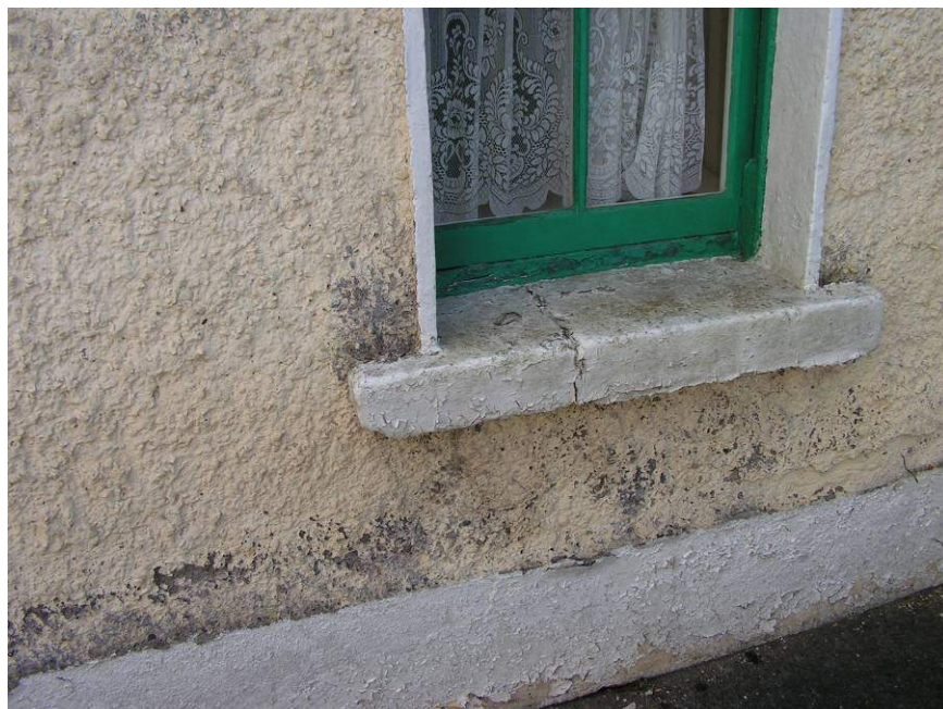
Fig. 8.3. A cracked and broken cill in number 3 Millview Terrace. The cause of the crack is not yet understood. (May 2011)
