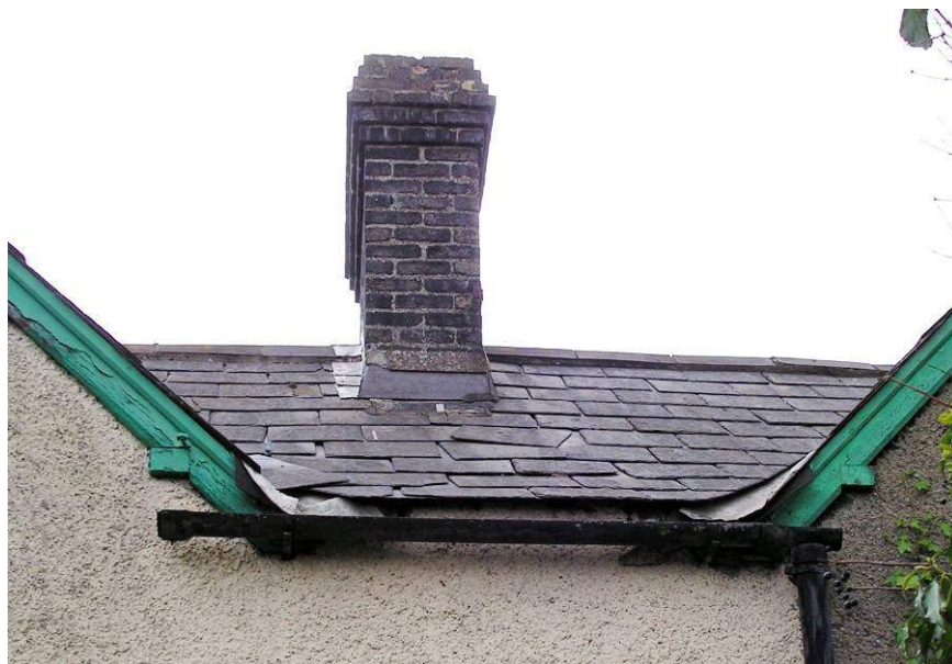
Fig. 7.8. Slipped slates above numbers 2 and 3 Millview. Note also the decay in the verge, the eroded flaunching mortar at the top of the chimney and the absence of any chimney pots. (May 2011)
