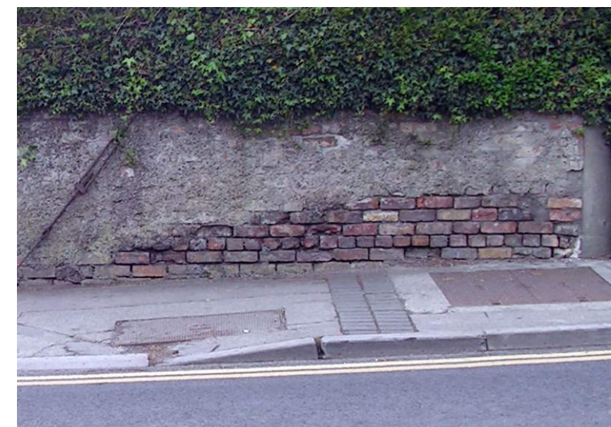
Fig. 11.1. The front boundary wall of number 3 Millview to the old Nangor Road. The brick wall urgently needs to be re-pointed. (May 2011)
