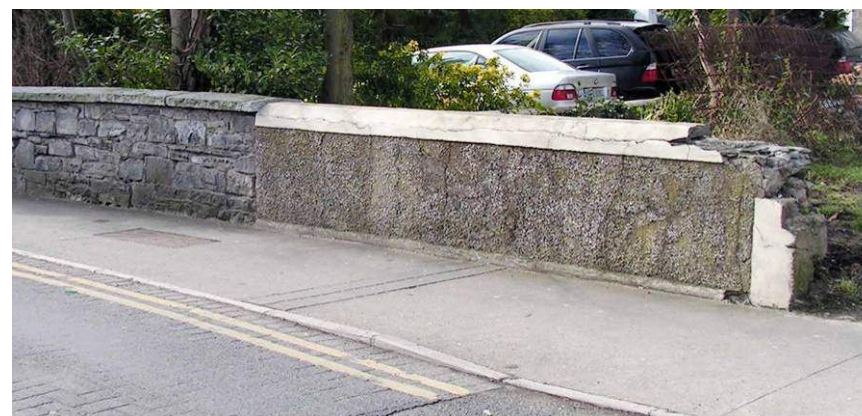
Fig. 3.10. Part of the former boundary wall of Moyle Park estate along Convent Road. The wall has had its coping removed, been reduced in height, punctured to give access to driveways, and in places rendered.
