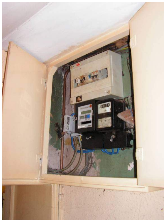
Fig. 7.15. The electrical circuit board in number 3 Millview. (May 2011)
