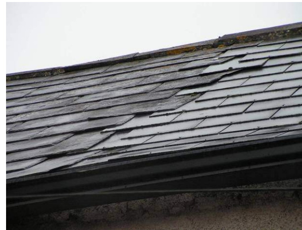
Fig. 6.11. Slipped and missing slates at the junction of the natural slates above number 16 and artificial slates of number 15. (January 2013)
