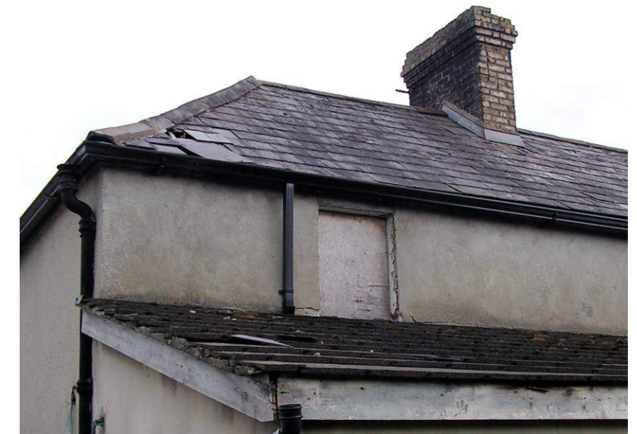
Fig. 7.1. Breaches in the roofs above 16 Tower Road, partly missing gutter, and decay in the fascia and soffit above the extension (May 2013)
