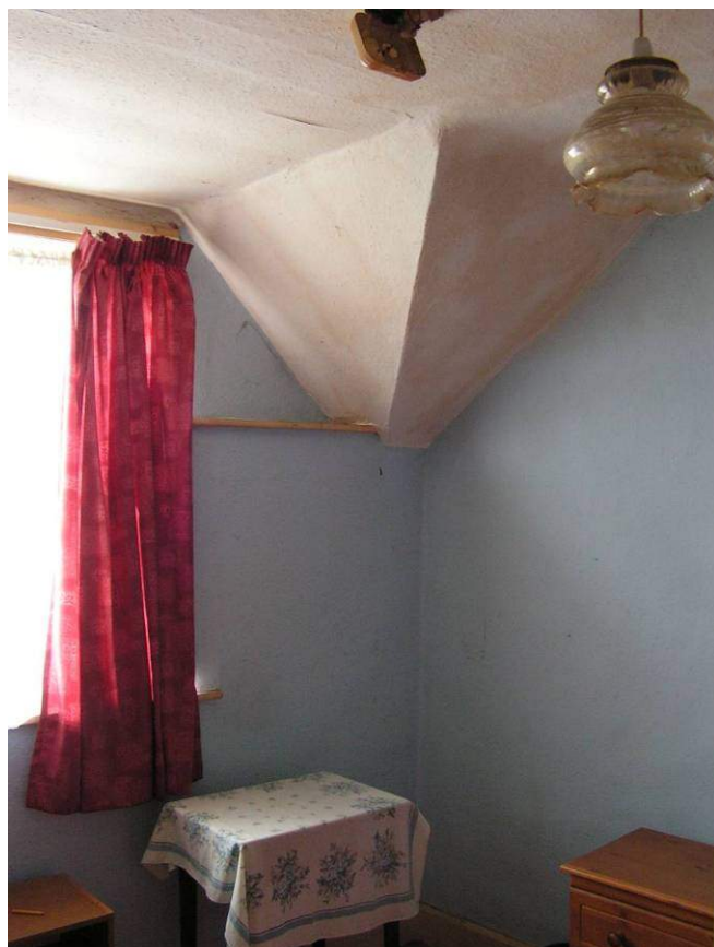
Fig. 11.6. Stained plaster and peeling wallpaper as a result of water ingress from above, first floor level number 3 Millview. (May 2011)
