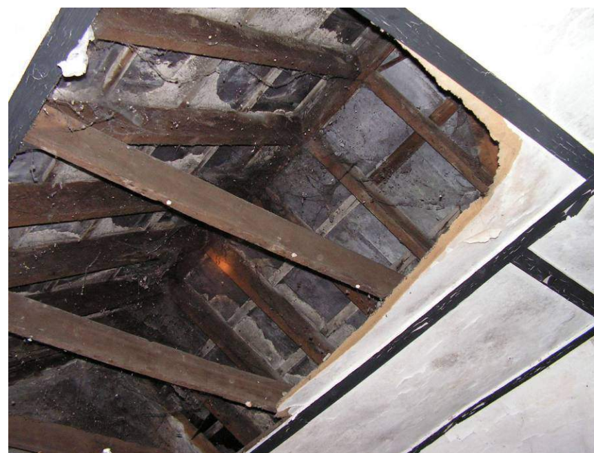
Fig. 11.7. Failure of the ceiling in 2 Millview Terrace. The parging mortar on the undersides of the slates above has also failed. (March 2013)
