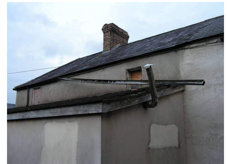
Fig. 7.2. Fallen gutter at the back of 16 Tower Road. (November 2013)
