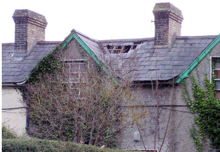
Fig. 7.3. Breaches in the roof of number 2 Millview and several slipped slates. Note also the extensive colonisation of the wall and part of the roof by ivy. (November 2013)
