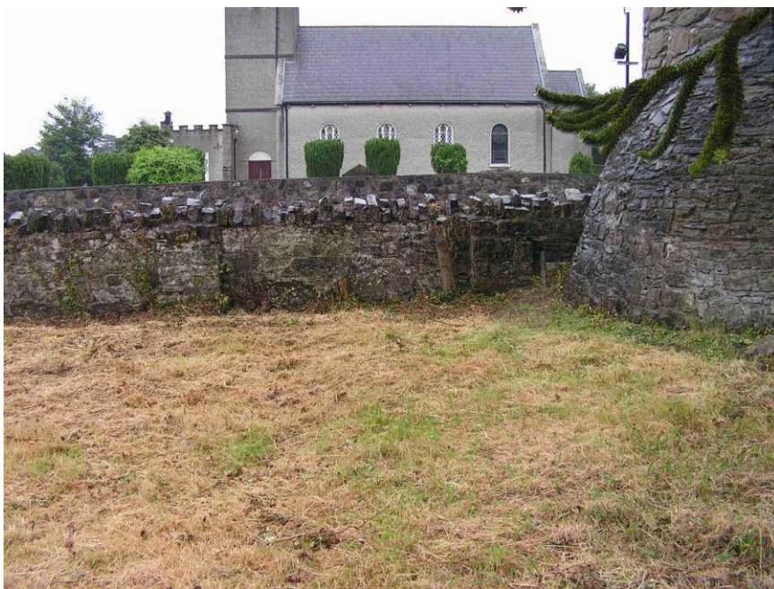
Fig. 11.2. The stone boundary wall along Tower Road just to the north of the round tower. Note the remains of a building. (June 2013)
