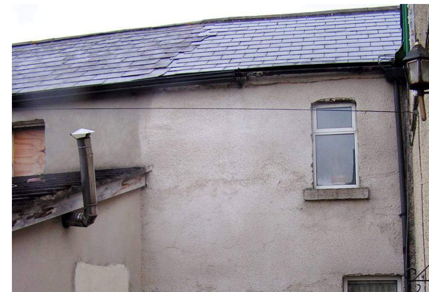
Fig. 11.4. Biofilms on the render at the back of numbers 15 and 16. Note also the missing gutter, the decayed timber on the left foreground and the crude openings made in the back of the houses. Number 16 (left) is roofed with natural slate, number 15 with artificial fibre cement slates. The latter should be included in an asbestos survey. (January 2013)
