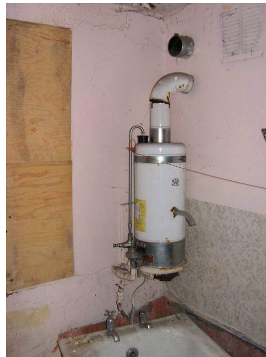
Fig. 7.16. A water heater and bath in the rere extension of 2 Millview Terrace. (March 2013)
