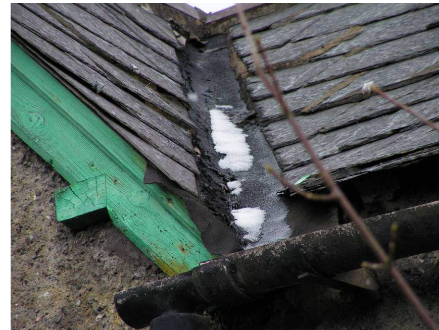
Fig. 7.7. 2 Millview Terrace. The lead has been stripped from the valleys where the dormer roofs join the main roof (March 2013)
